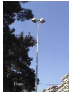
Typical street light in Plastira street
